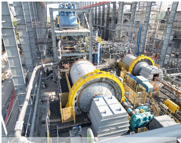
Beneficiation Plant at Dariba, Rajasthan
