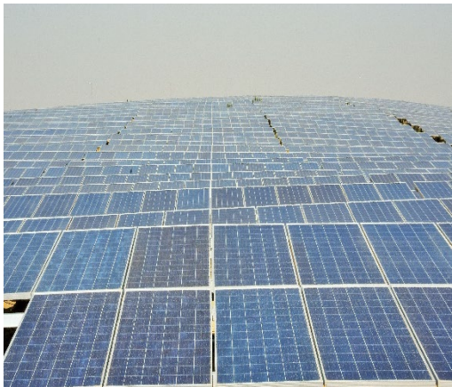
150 MWp Ground Mount Solar Project, Rajasthan
