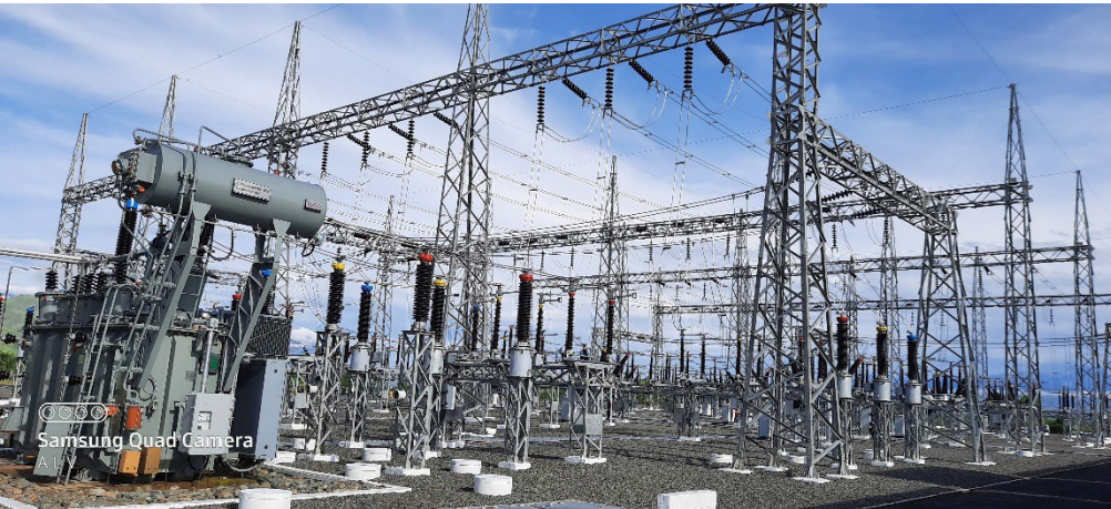
132 kV Air Insulated Substation, Papua New Guinea
