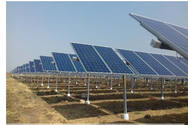
30 MW Tracker Based Installation, Andhra Pradesh
