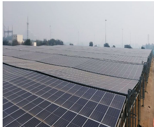
20 MW Solar Carport project, Haryana
