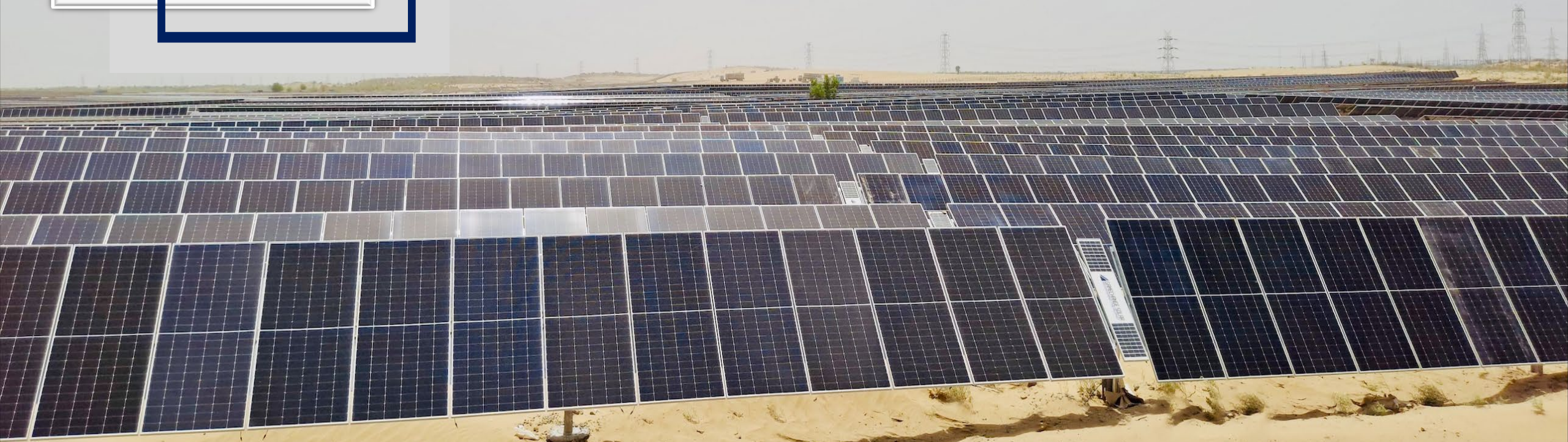
500 MW Solar Project at Bhadla, Rajasthan
